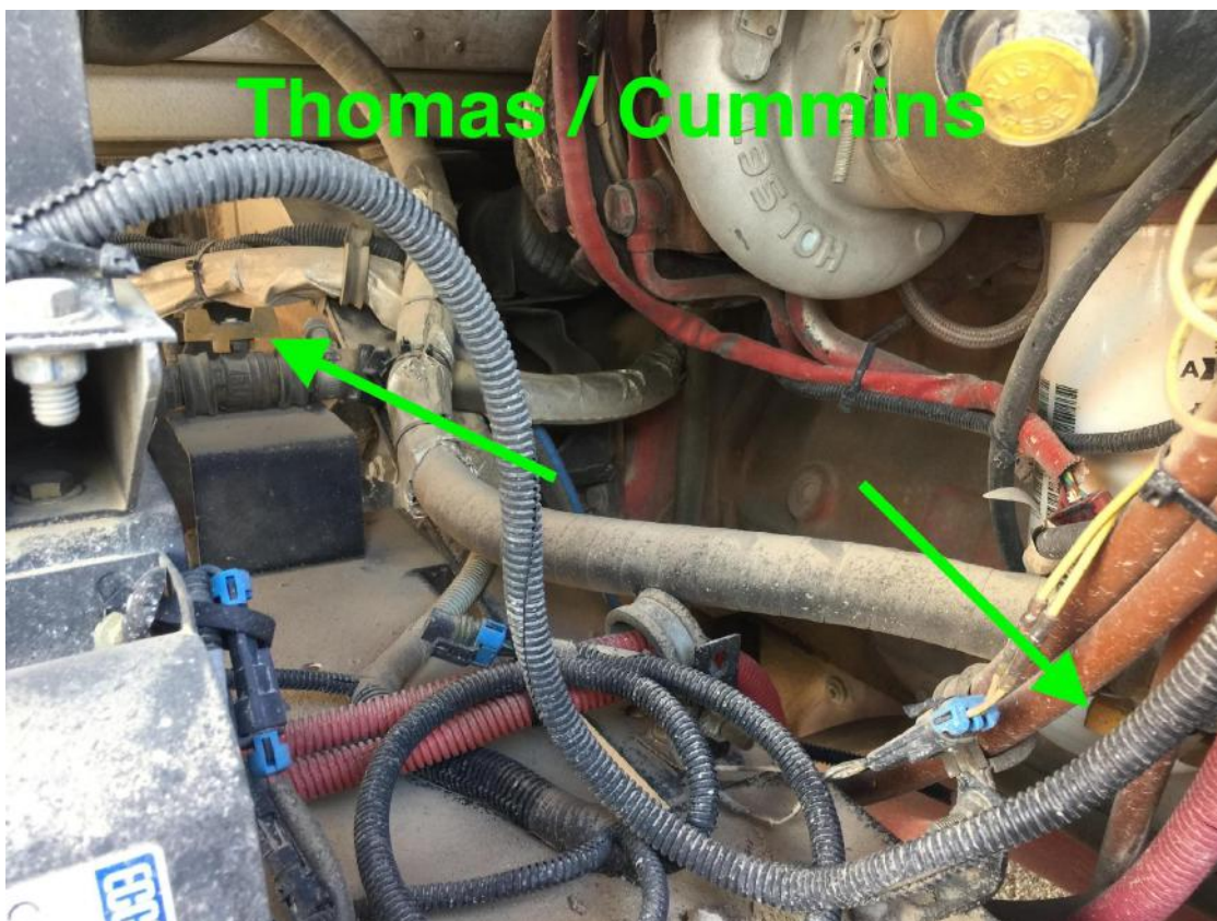
Figure 12 – Thomas Cummins Heater Valves
